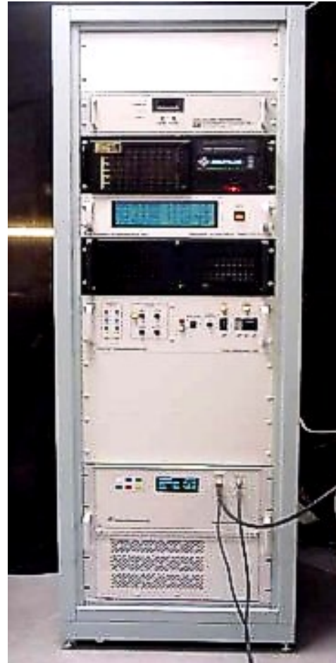
RVP8 Installed In Radar System Cabinet
